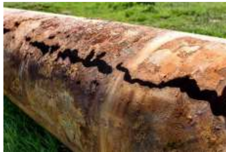
Figure 1. Corroded Pipeline Courtesy: google
