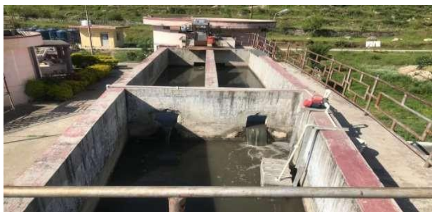
Fig.8 inlet from where the wastewater taken before the treatment of wastewater
