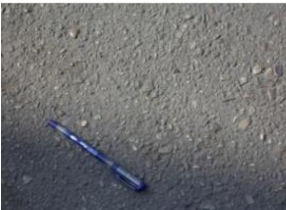
Figure 12. Pavement surface in A
