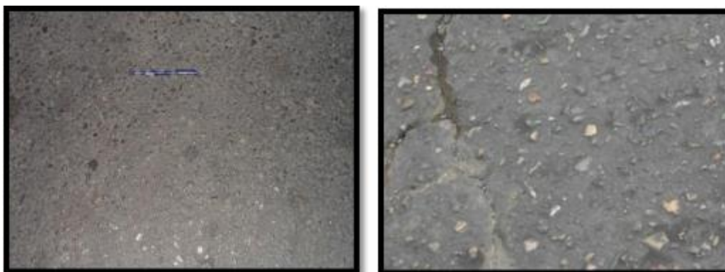
Figure 9. Damage to the pavement Surface
