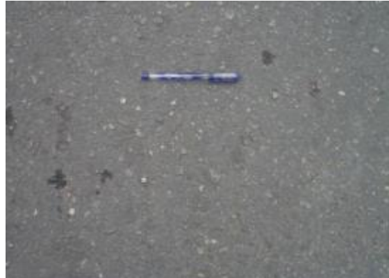
Figure 17. Pavement surface in F
