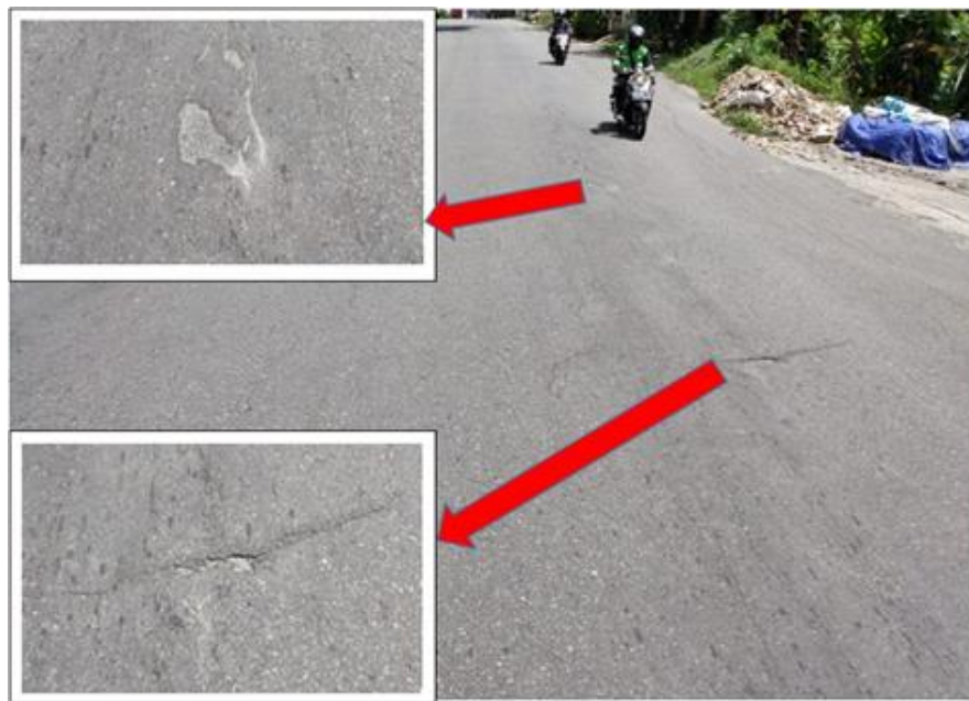
Figure 2 Condition of Cracks and Holes on J. Syaranamual Street
