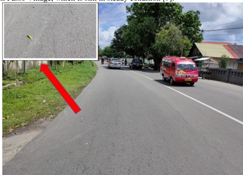
Figure 3 Condition of Cracks on Laksdya Leo Wattimena Street
