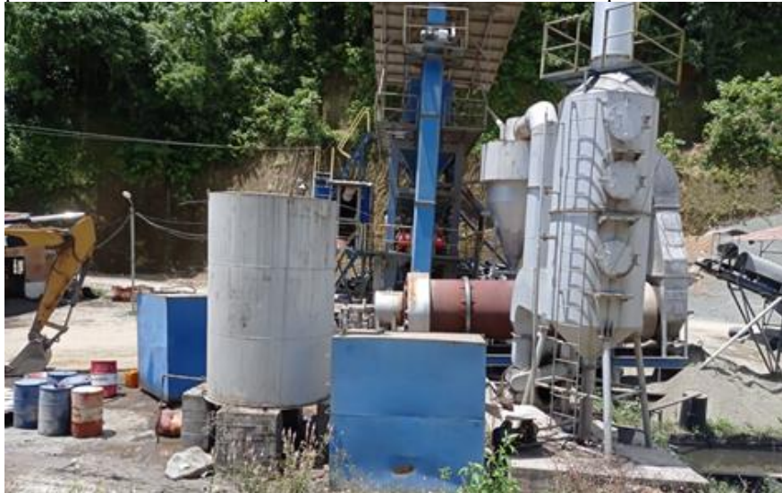
Figure 5 Asphalt Mixing Plant (AMP) in Laha Village-Ambon
