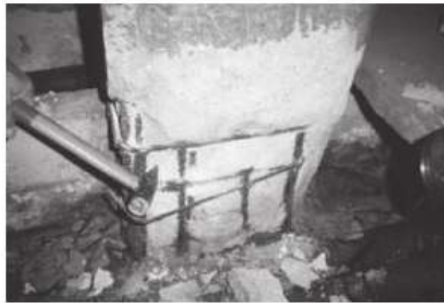
Figure 1. 4 a column steel reinforcement bars after 10 years exposed within a closer area
