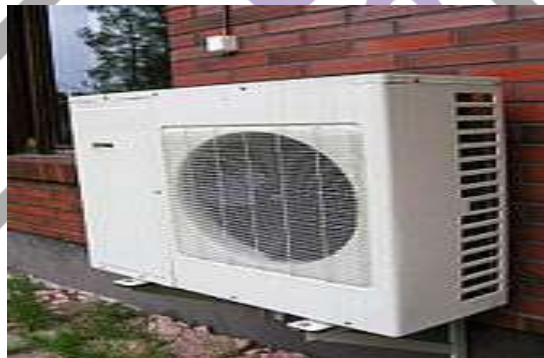
Figure 1.2: Externally fitted AC unit with heat pump
