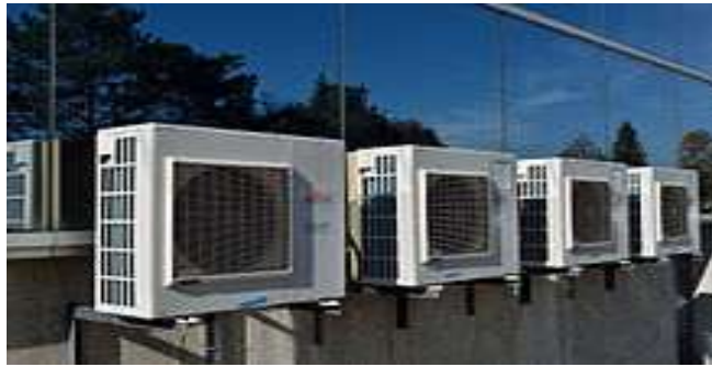
Figure 1.4.1.1 an array of air conditioner outdoor units
