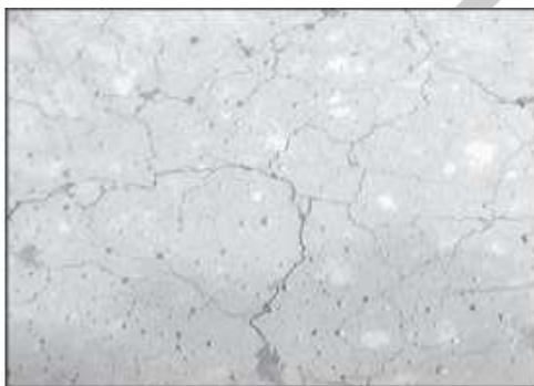
Surface cracking after subject to high temperatures.
