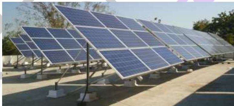
Fig.2.50 kWp solar PV plant
