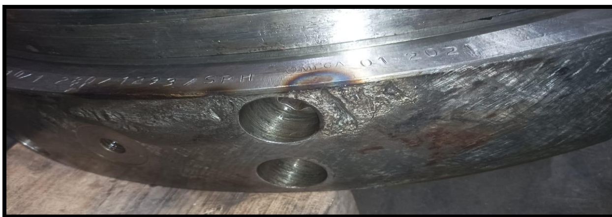
Figure 6: Discharge evidence at torus contact surface.
